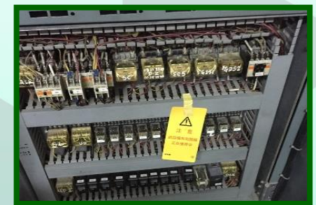
Figure 3 (8.1.c.v): Display the warning sign at controller and the place where the inspection mode can be shifted
