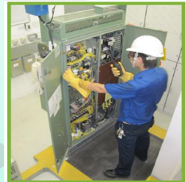
Figure 14 (8.8.5d): Lift workers should use suitable PPE with electrical insulated gloves / shoes and stand on an insulation mat when working on live electrical equipment
